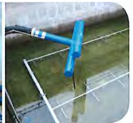
Fixed Diffused Aeration
