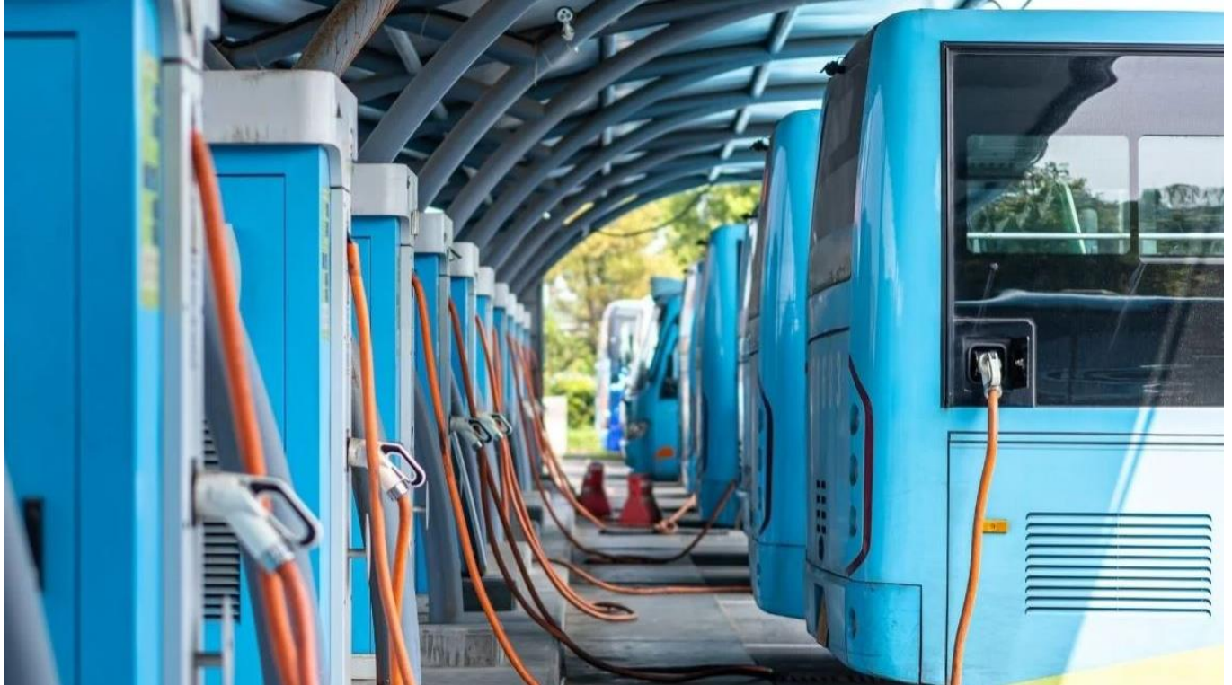
Figure 9: Plug-in Bus Depot Chargers
