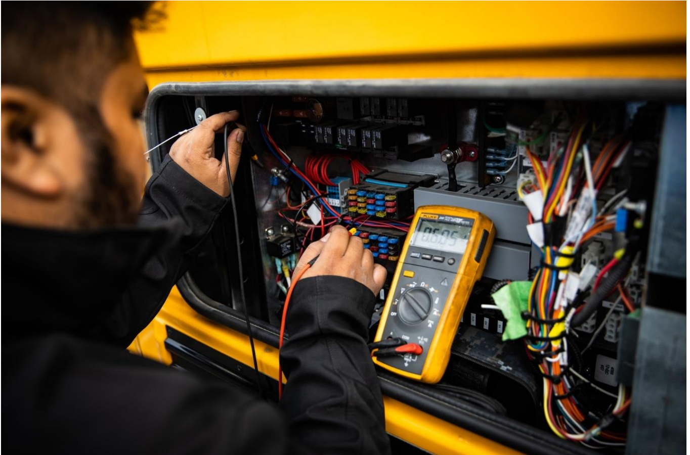
Figure 11: BEB Technician Utilizing a Multimeter
