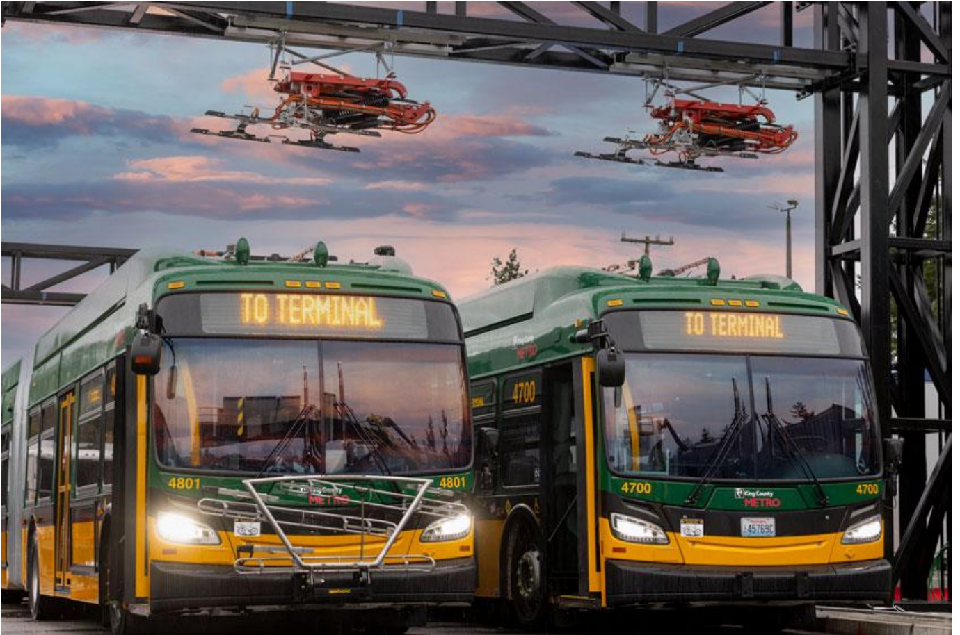
Figure 10: King County Metro Pantograph Chargers at Bus Depot
