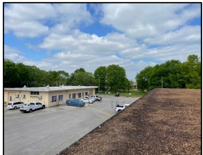
Figure 4-8: “PPD” West-Facing View
