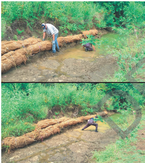
Figure 4. Placing and anchoring cedar revetments for streambank stabilization in Lytle Creek, August 2018.
