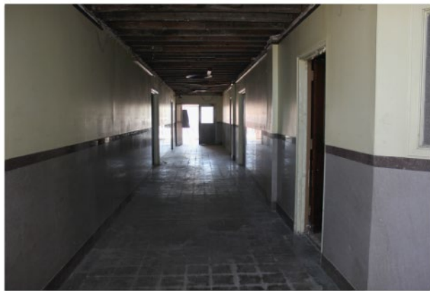
Photo 21 Universal Life Insurance Company 7/31/15 View from the rear entrance door looking along the central axial corridor to the front door.
