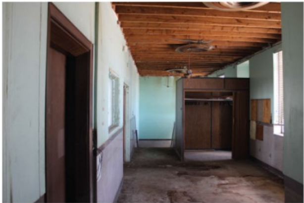
Photo 24 Universal Life Insurance Company 7/31/15 View of the second floor public lobby, looking towards the stair to the first floor.
