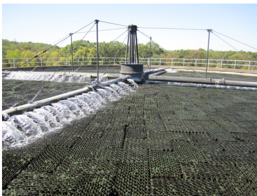
Columbia WWTP - Nitrification Tower
