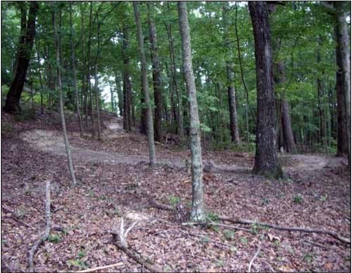
SORBA Chattanooga trail construction project at TVA’s Raccoon Mountain facility. Flowing turn with out sloping trail and reverse grade water dips.
