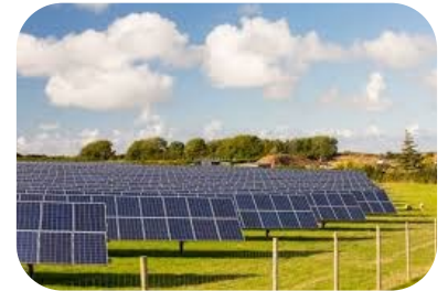
Renewable Energy Generation
