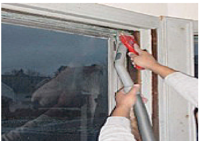
FIGURE 11.12 Vacuum window again.
