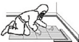
FIGURE 12.10 Install underlayment and new flooring as a suitable LBP enclosure method. The personal protective equipment is for a high-dust project.
