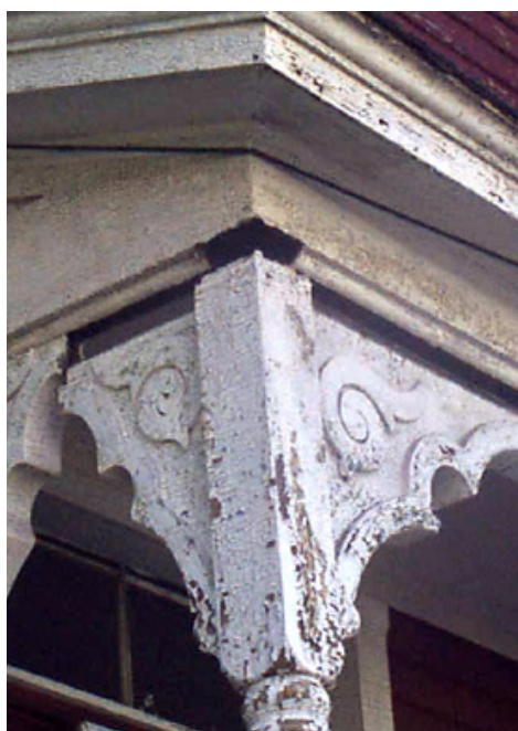
FIGURE 1.2 Deteriorated residential paint on house trim.
