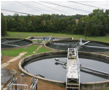
Trickling Filter/Solids Contact
