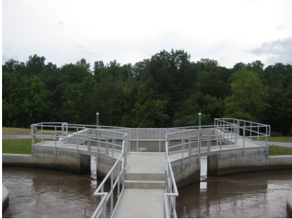
Anaerobic Selector for Phosphorus removal
