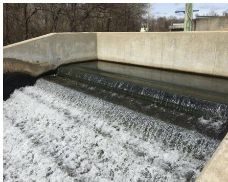
foam in effluent (at cascading outfall) due to coagulant/polymer (added for PO 4 removal)
