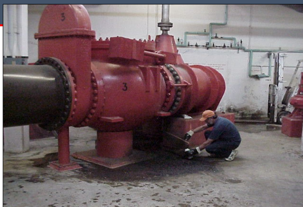
Return Activated Sludge Systems
