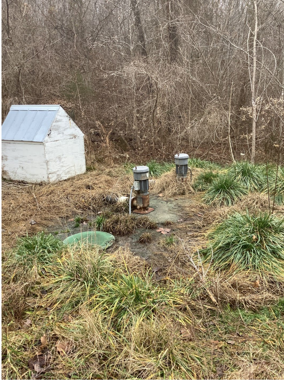
X2. Wastewater effluent being discharged from the pump vaults rather than to the drip field.
