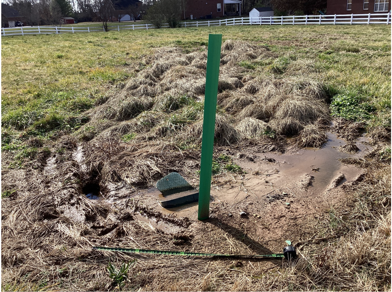
X3. Infrastructure piping failure allowing extensive effluent release.
