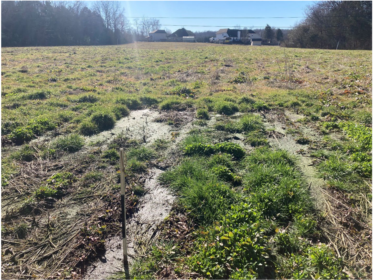
A2b. Extensive saturation/ponding.
