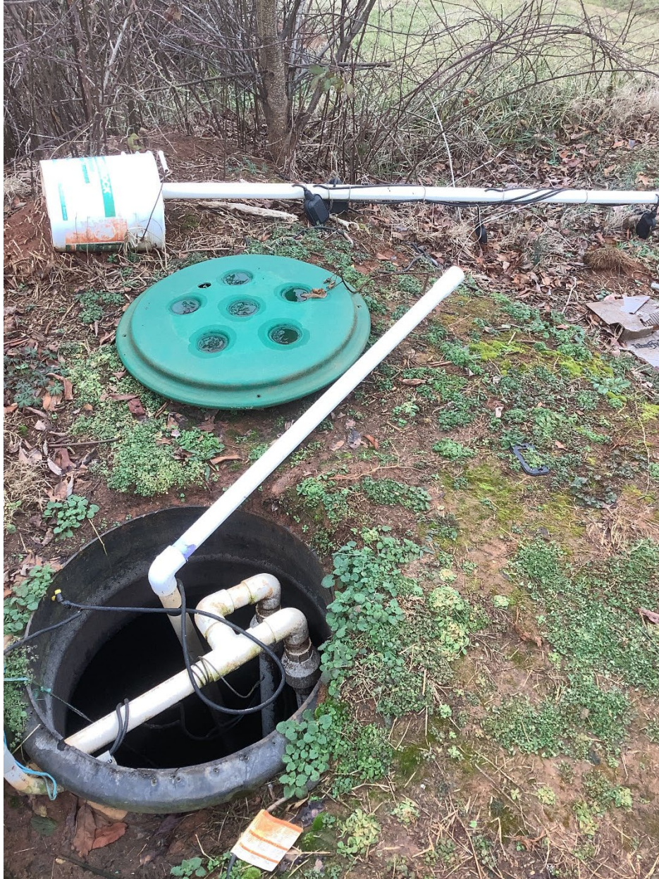
X2. Wastewater effluent being directed to adjacent ditch rather than the drip field.
