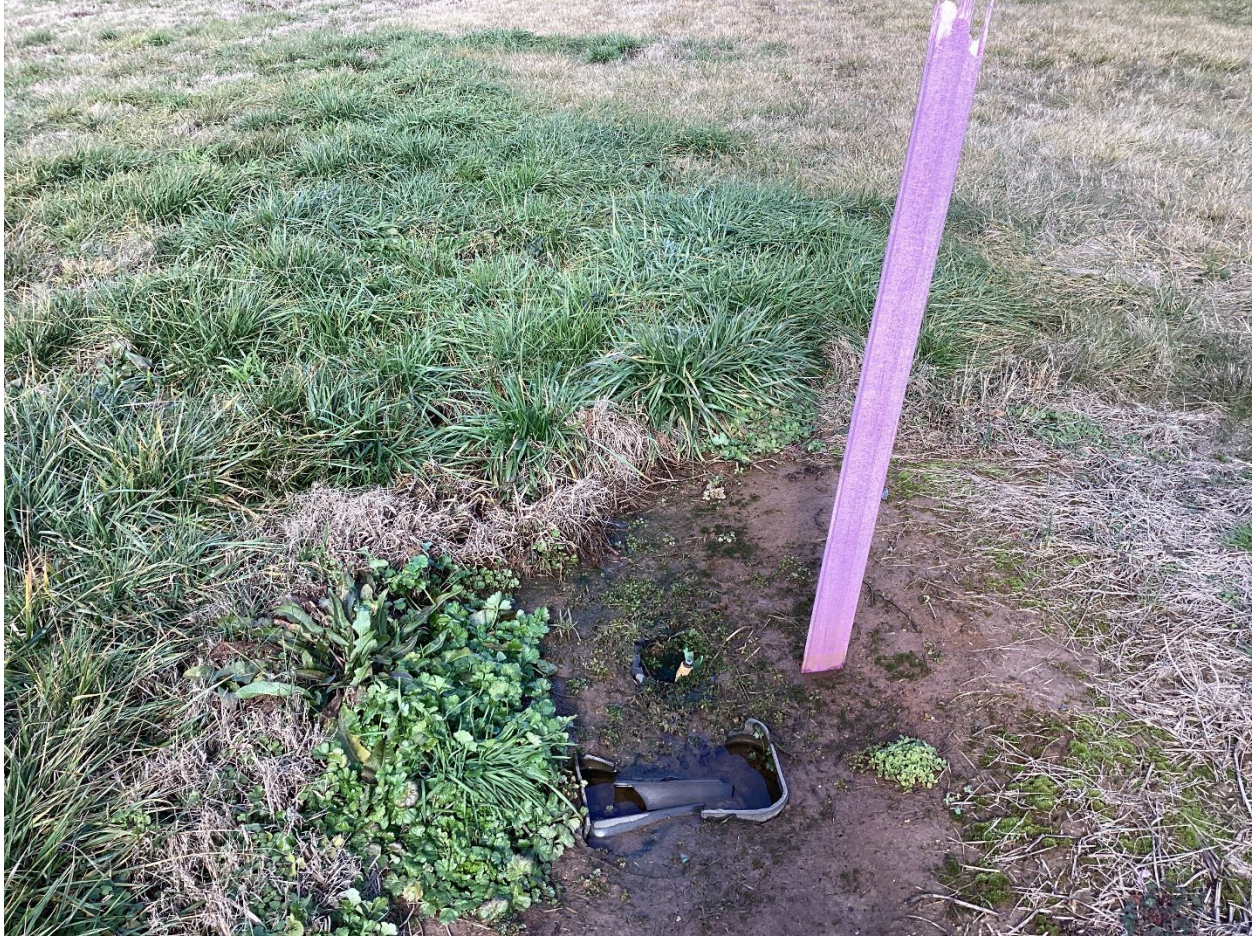
A2a. Localized saturation/ponding. Likely associated with a damaged valve.
