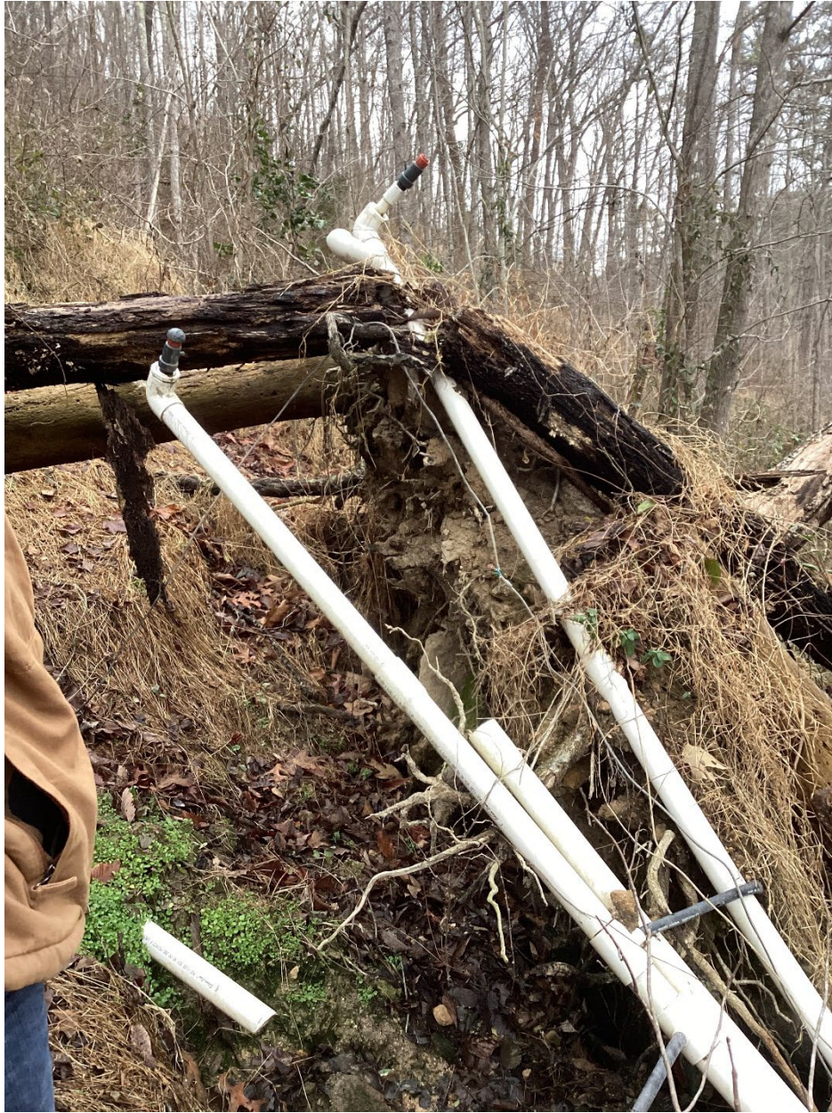
X3. Infrastructure piping unearthed and disconnected by uprooted tree.
