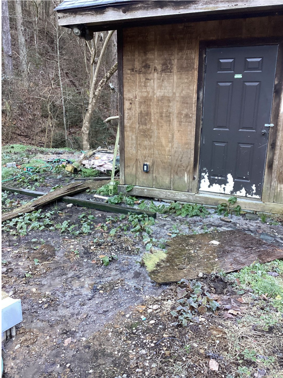
X2. Wastewater effluent being discharged from the control building rather than to the drip field.
