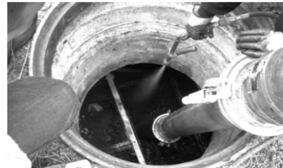
2. Insert vacuum hose in the sedimentation chamber and vacuum out all trash, sediment and standing water.
