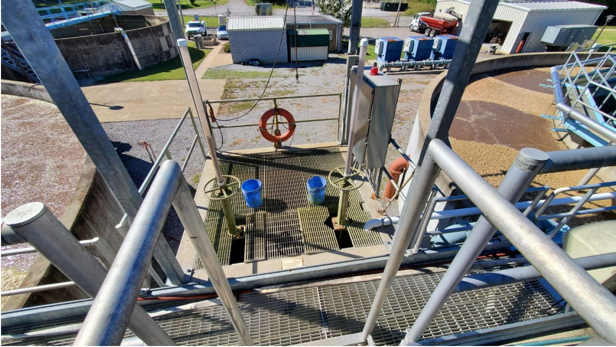
Influent Splitter Box with RAS.
