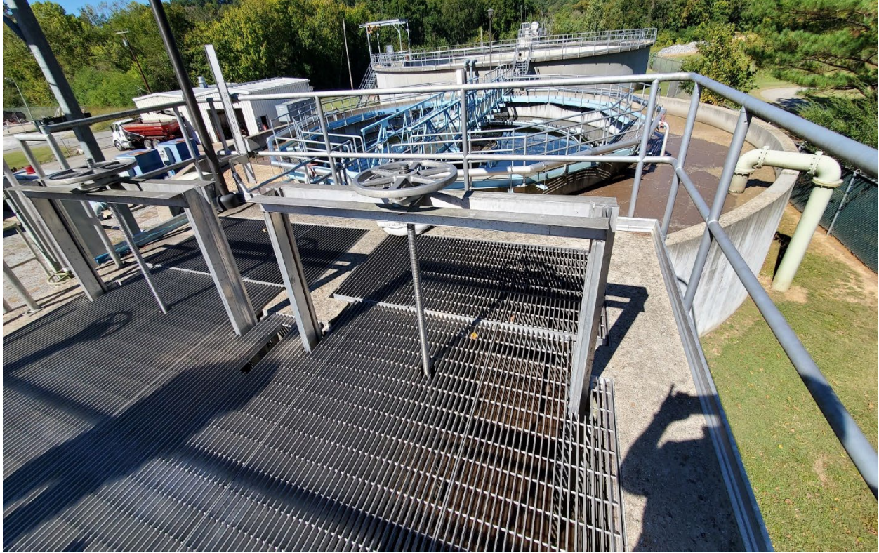
Aeration Reactor (2) with EQ Basin in background.
