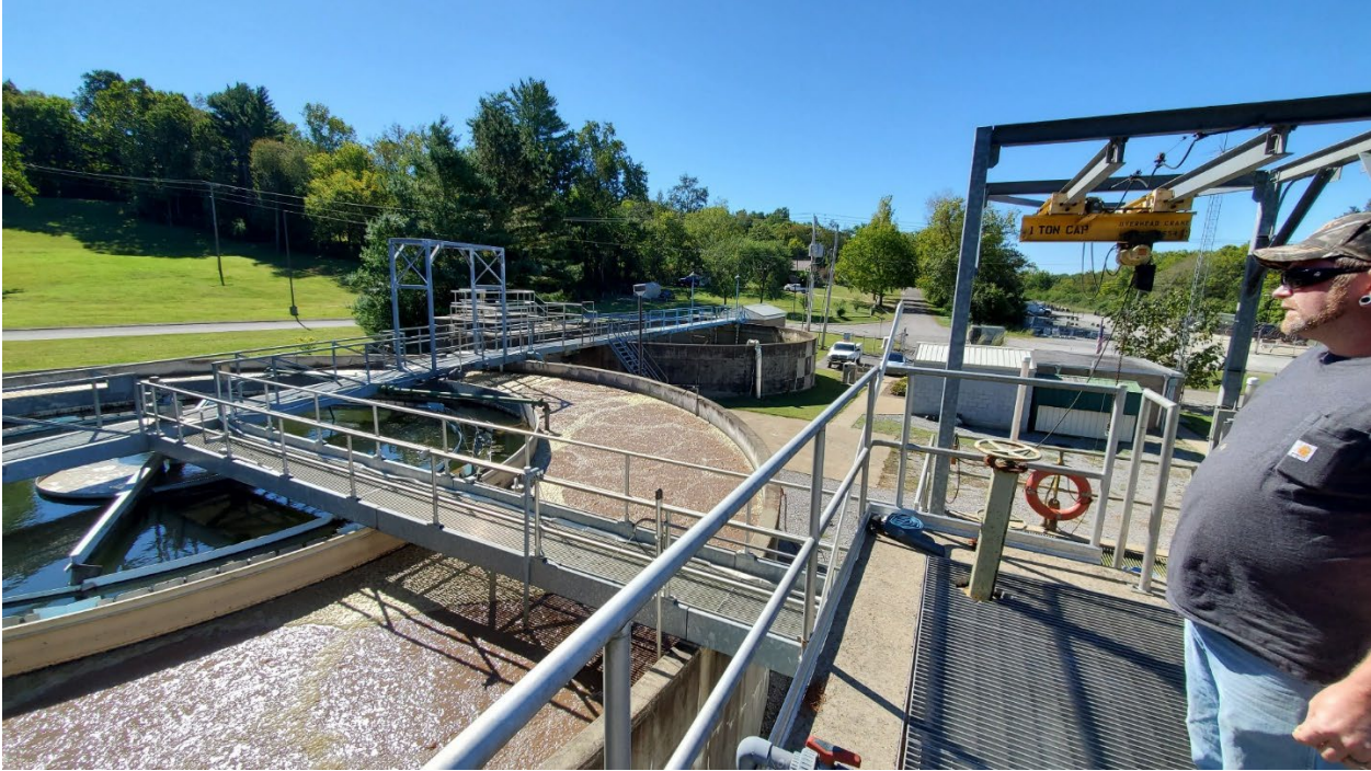
Aeration Reactor (1) with Center Clarifier Unit.
