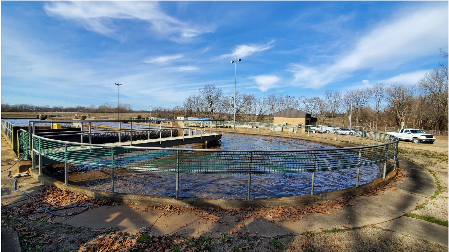
Dyer Oxidation Ditch – East Rotor
