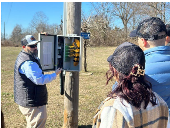
CABINETS ALONG THE NEW ROUTE.
