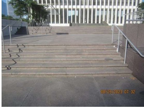
Overview of the stair where transitions are anticipated to occur in the below waterproofing system.
