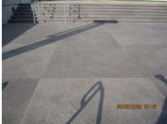
Overview of the area where a drain system has been covered. NRC recommends removing the finish components above the drainage system to promote observation of the drainage relief point.
