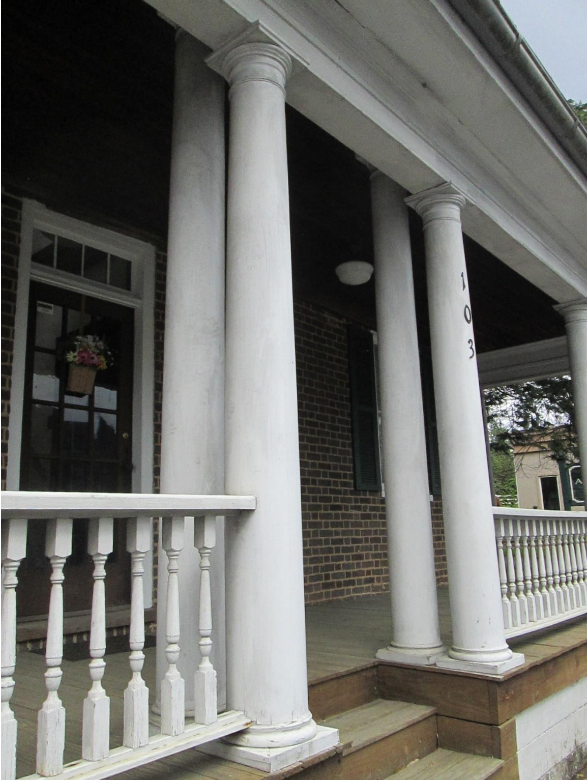
Photograph 8. Examples of the freestanding columns along the east elevation (façade) of the Nance Building, shown in fair condition.
