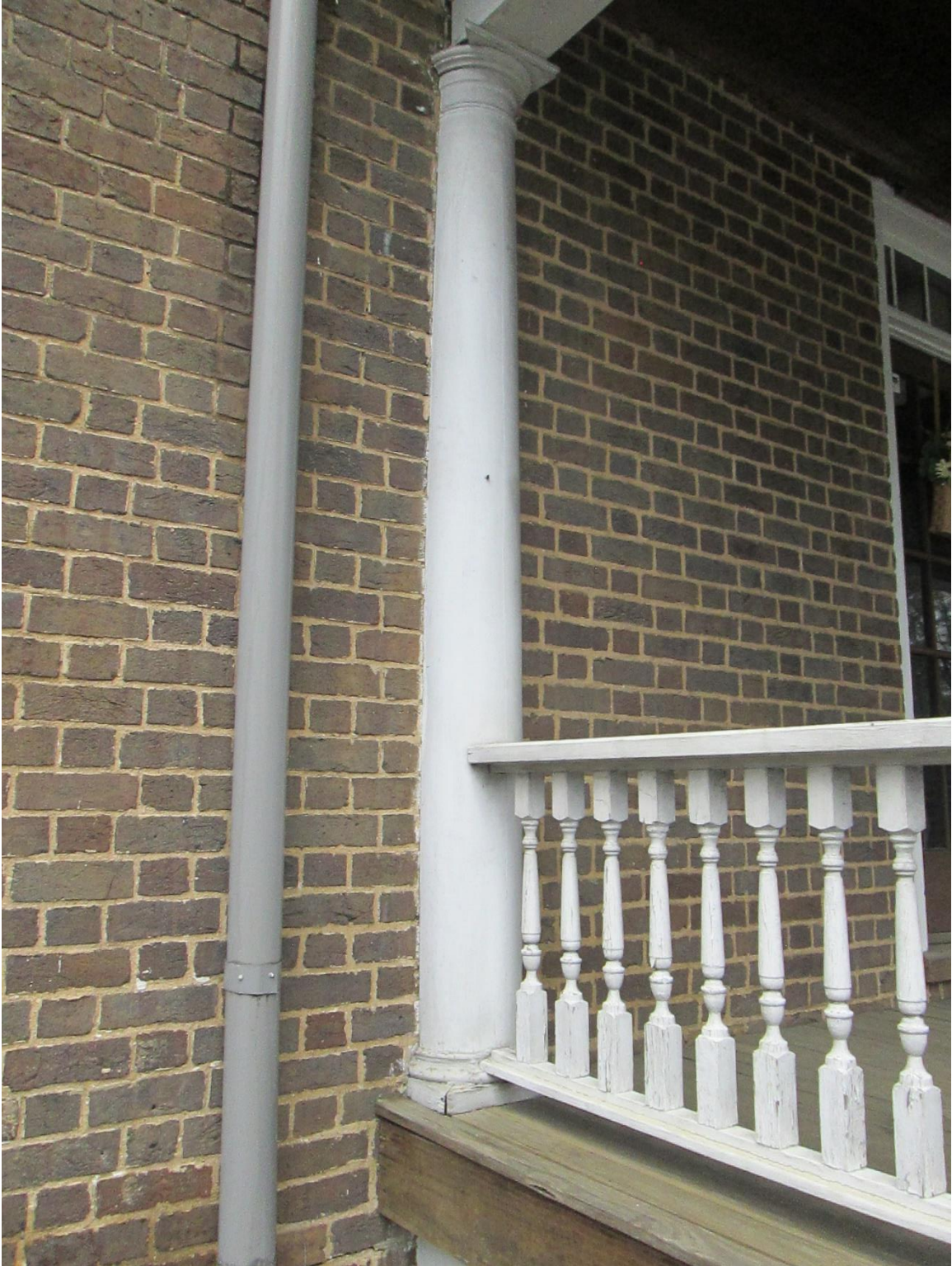
Photograph 9. Example a pilaster along the east elevation (façade) of the Nance Building, shown in fair condition.
