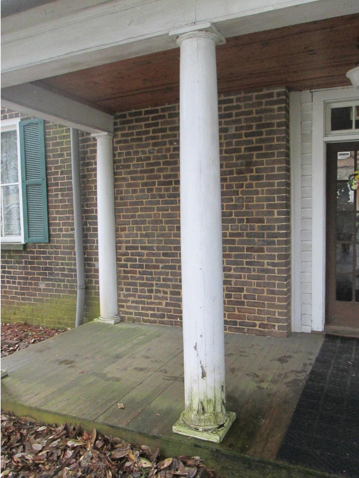
Photograph 5. Example of moderate deterioration of a freestanding column along the north elevation of the Nance Building
