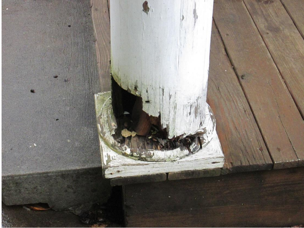
Photograph 2. Example of substantial deterioration of a freestanding column along the west elevation of the Nance Building.
