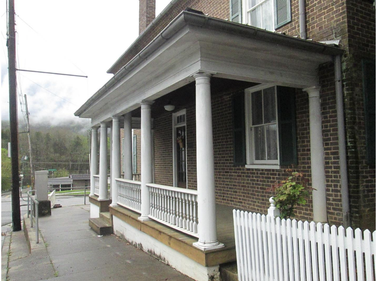
Photograph 7. Partial view of the east elevation (façade) of the Nance Building, facing southwest, showing the entire porch including the seven freestanding columns and two pilasters.
