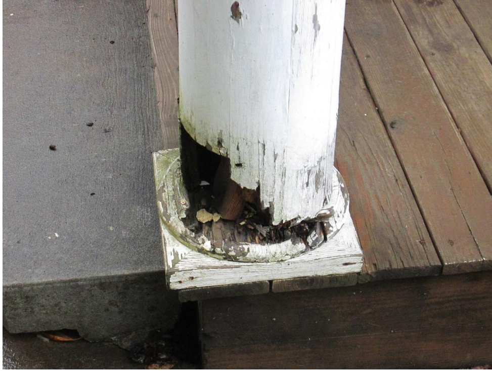
Photograph 2. Example of substantial deterioration of a freestanding column along the west elevation of the Nance Building.
