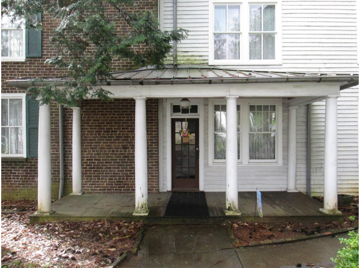
Photograph 4. Partial view of the north elevation of the Nance Building, facing south, showing the entire porch including the four freestanding columns and two pilasters.
