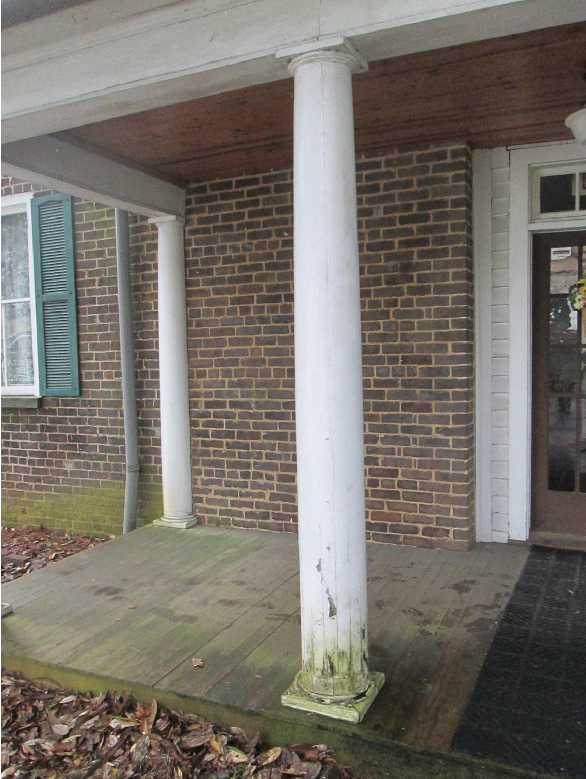
Photograph 5. Example of moderate deterioration of a freestanding column along the north elevation of the Nance Building
