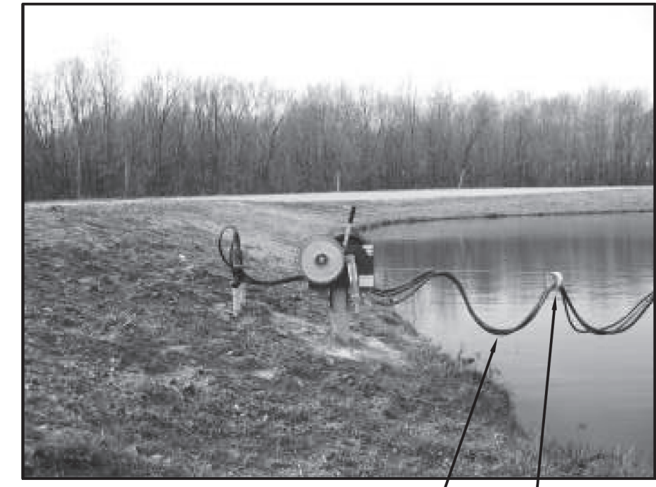
ELEC. CABLE SUSPENDED FROM ANCHOR CABLE CABLE LOOPS FABRICATED FROM SCHED 80 PVC CONDUIT
