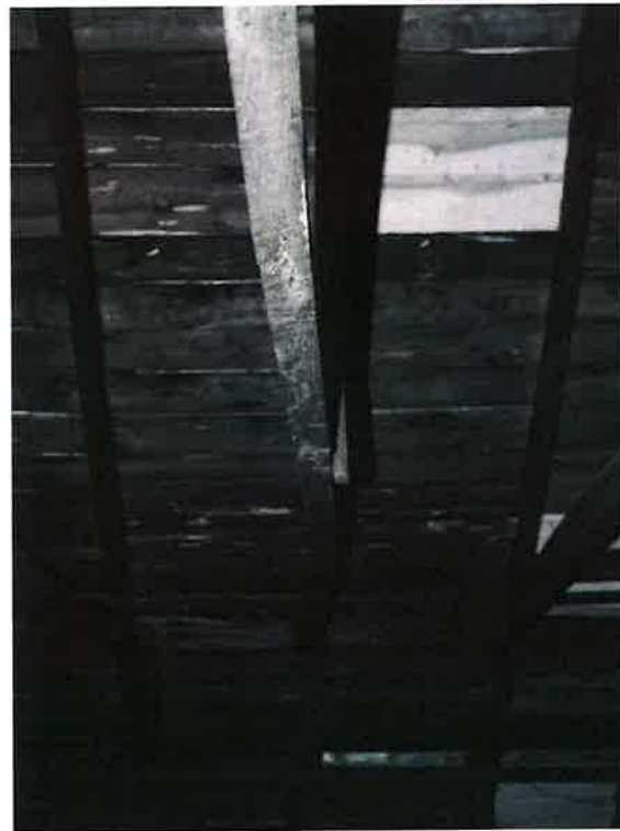
Photo No. 27. Warped bottom chord of roof trusses.
