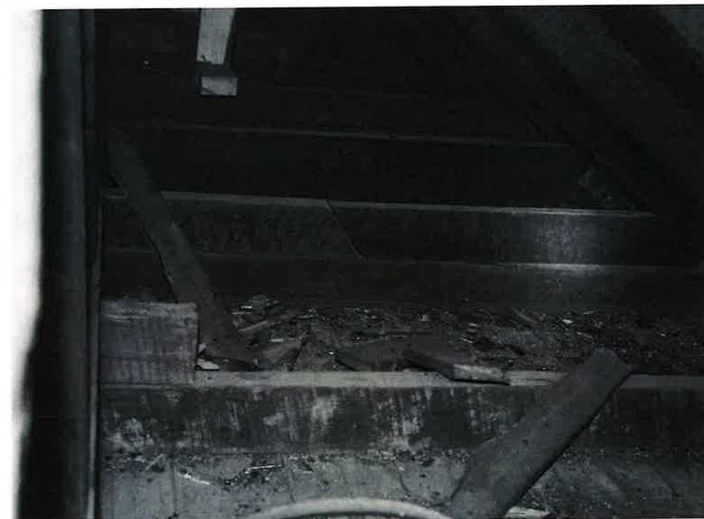
Photo No. 24. Porch ceiling framing with cracks at midspan.
