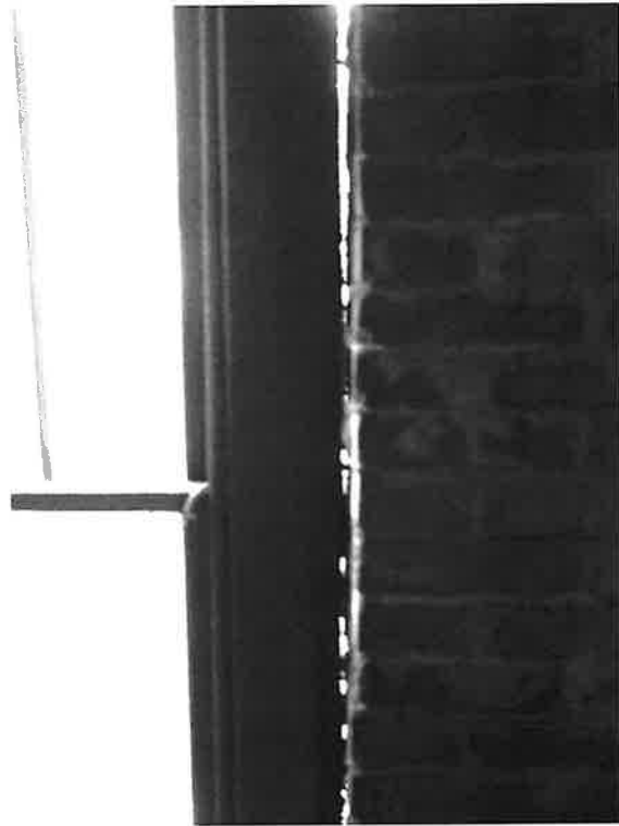
Photo No. 33. Typical gap around openings.
