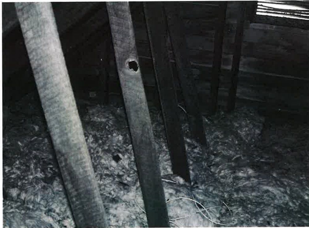
Photo No. 29. Typical warped truss webs above kitchen area.
