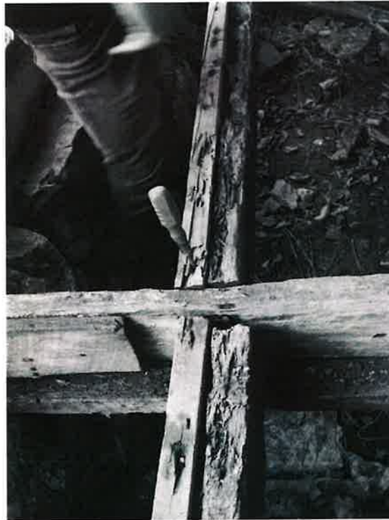
Photo No. 11. Section loss in front porch framing.
