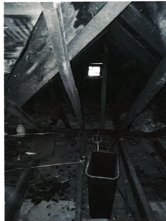
Photo No. 28. Warped top chord of roof truss near framing above kitchen.
