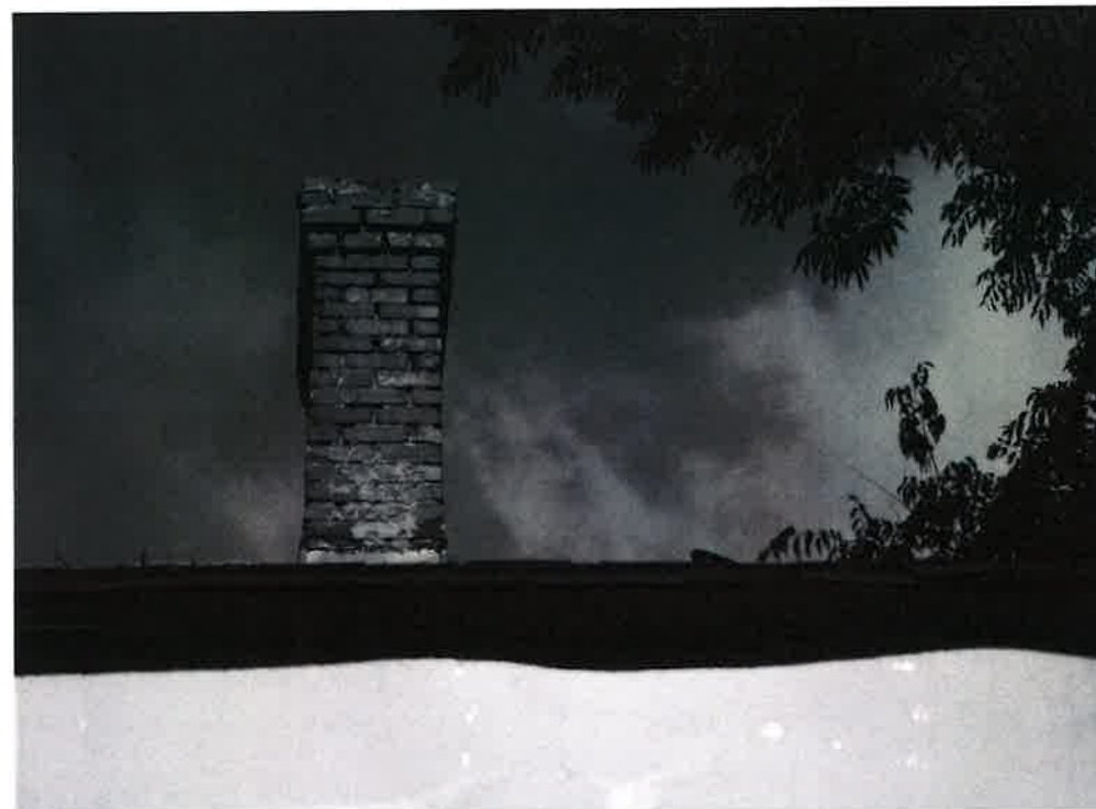
Photo No. 32. Brick chimney with mortar degradation.
