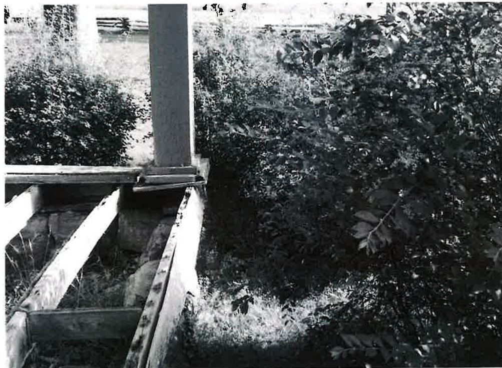
Photo No. 12. Improper supported column base.
