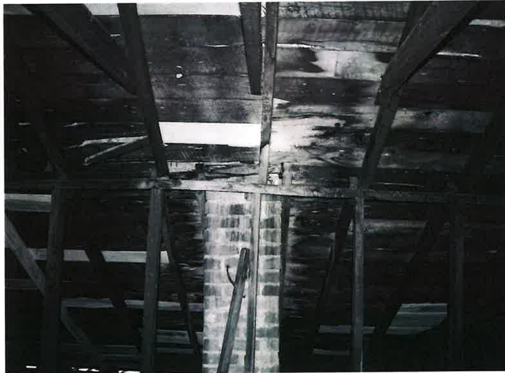
Photo No. 21. Water staining at current members with chimney penetration.
