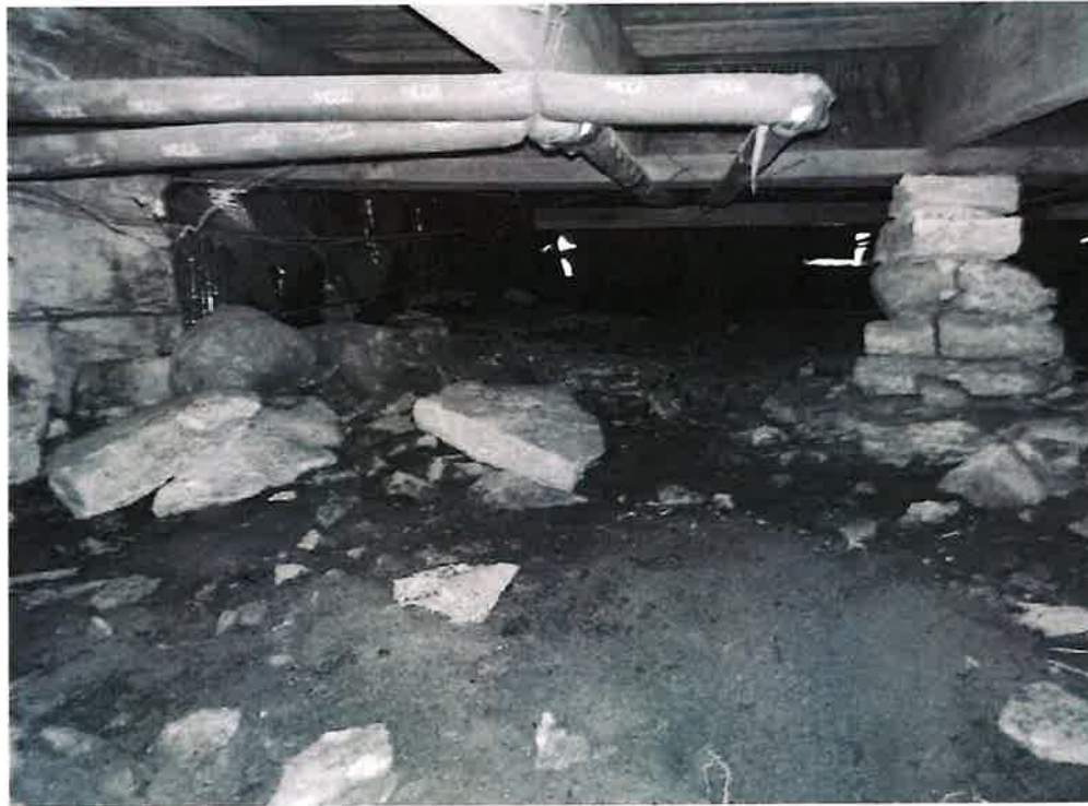
Photo No. 7. Stone pier that has fallen over.
