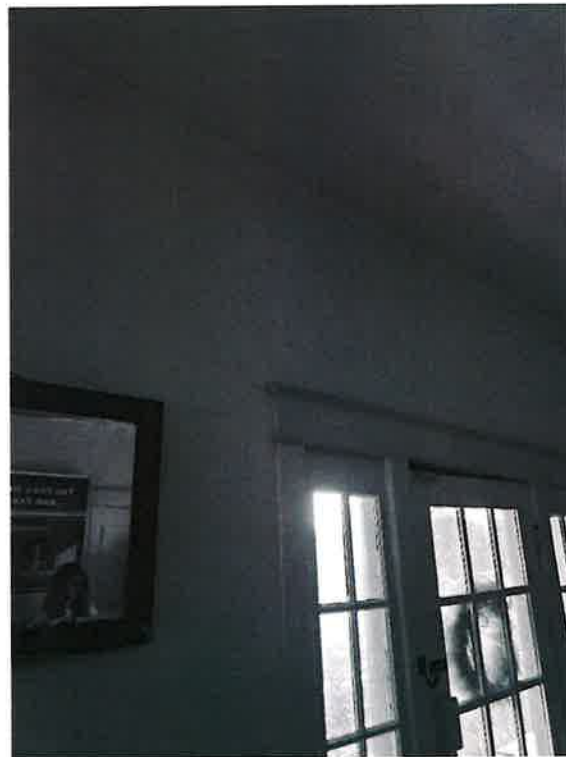
Photo No. 31. Crack in wall beneath attic.
