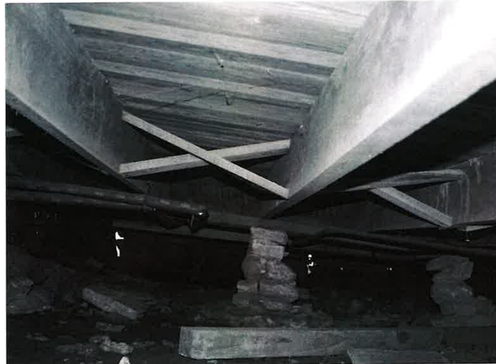
Photo No. 6. Stone pier with crack.
