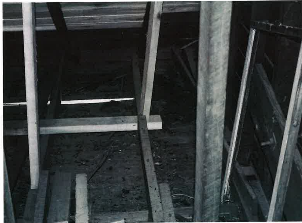
Photo No. 23. Porch ceiling framing changes size midspan.
