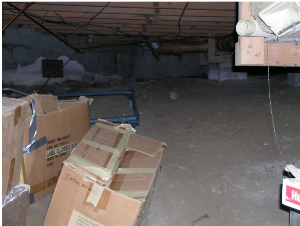
Photo 7 - View of the unfinished section of basement, essentially a crawl space, of Home B. There is storage of sealants, and paints in this area. (Photo credit: Joe George, TDH, 01/19/10).
