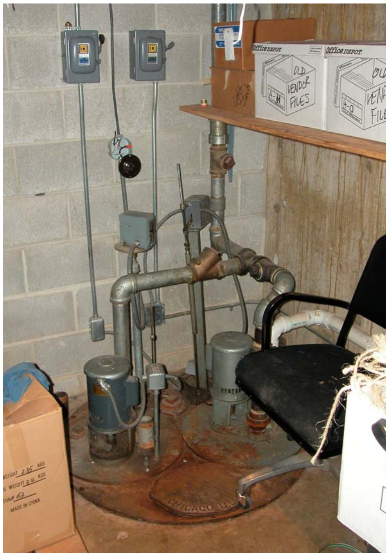
FIGURE 5 - The small basement storage room (indoor air sampling Station B) within the Bradford Building where a sump pump is located. Water samples were collected from this sump. (Photo credit: David Borowski, TDH, 12/20/04)
