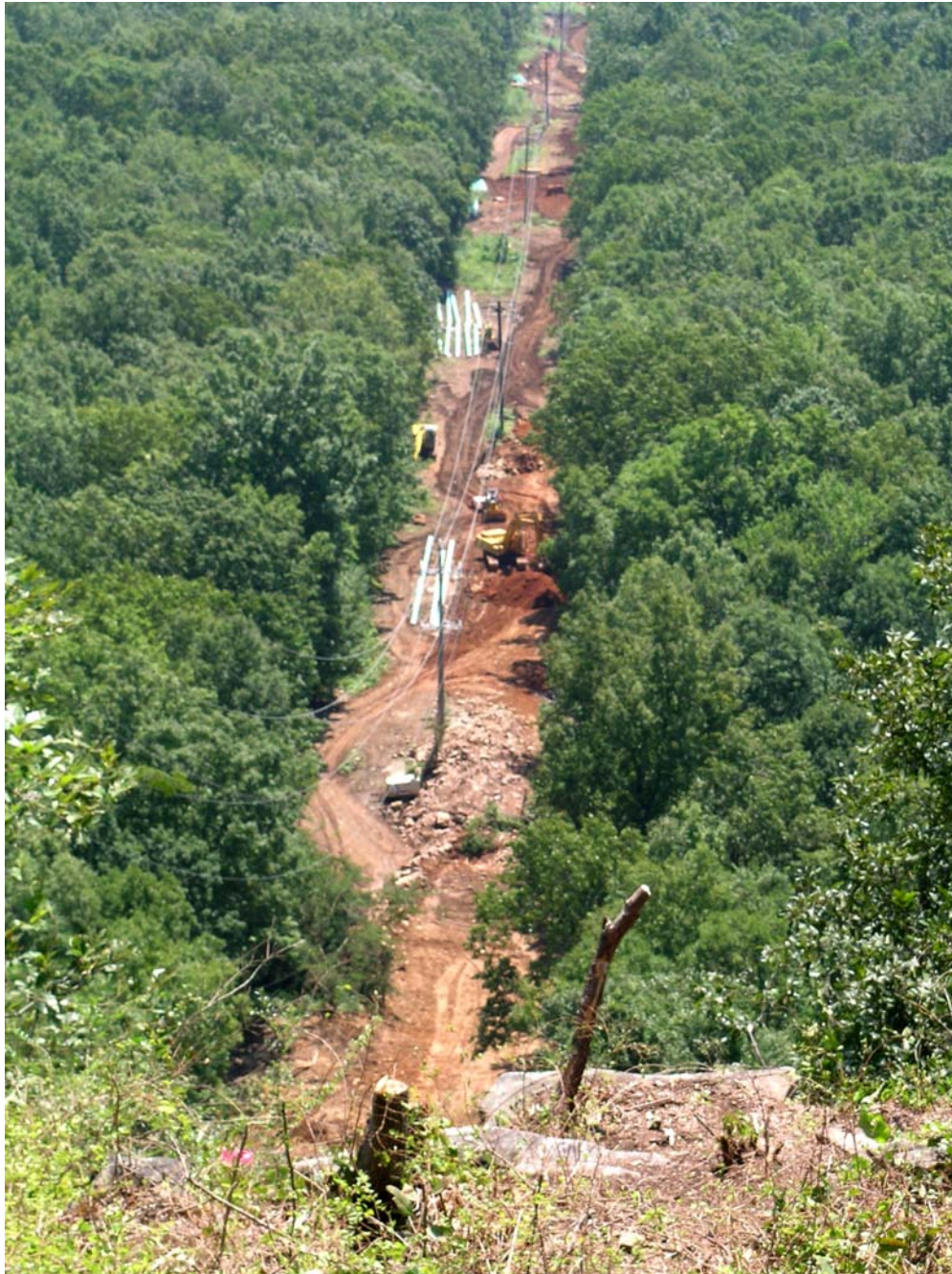
FIGURE 4 - Photo of the new water line construction. This view is looking to the east from the top of the Cumberland Escarpment (on East Brow Road). Walden, Hamilton County, Tennessee. (Photo credit: Ron Clendening, TDH, 8/31/05)
