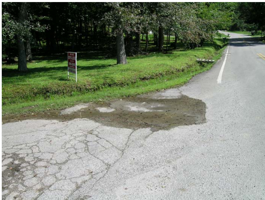
FIGURE 6 - Photo of water seeping from Timesville Road, at the intersection with Lewis Mine Road, in the Timesville community. (Photo credit: Ron Clendening, TDH, 8/31/05)
