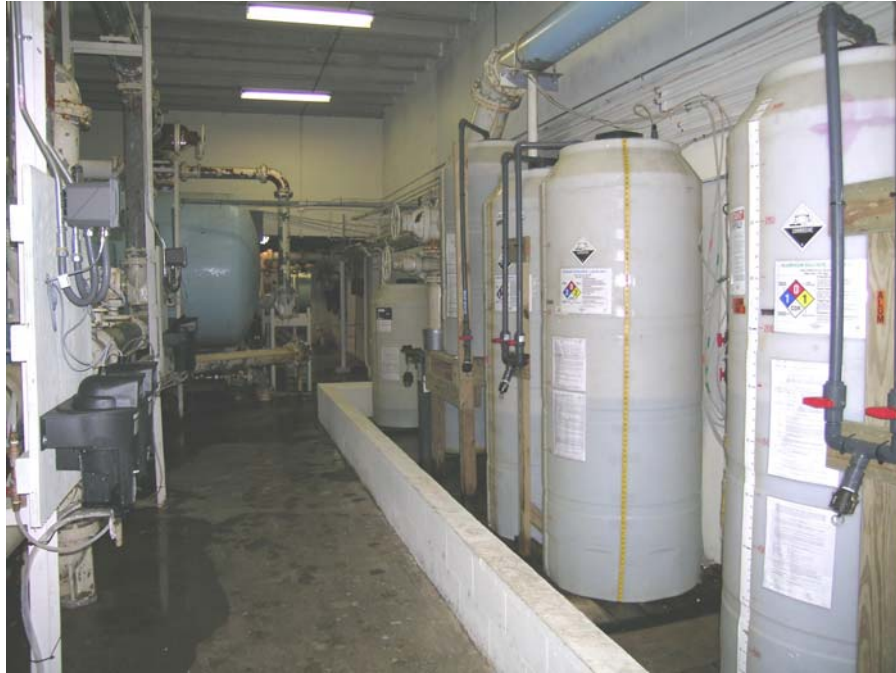
FIGURE 2 - Photo of the WRUD Water Treatment Facility. Hamilton County, Tennessee. (Photo credit: Ron Clendening, TDH, 8/31/05)
