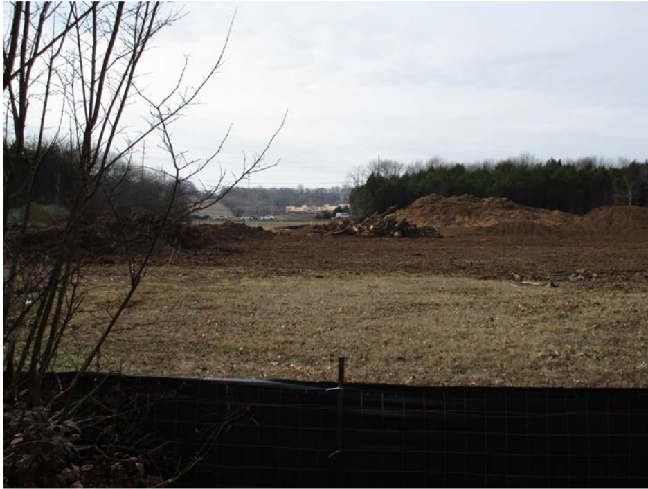
Figure 2. TDH photograph of the site taken January 16, 2017, after initial construction that shows piles of chipped materials after much of the woods and undergrowth was removed. The photograph was taken from Forest Pointe Place dead end looking west to Murfreesboro Road in the distance.
