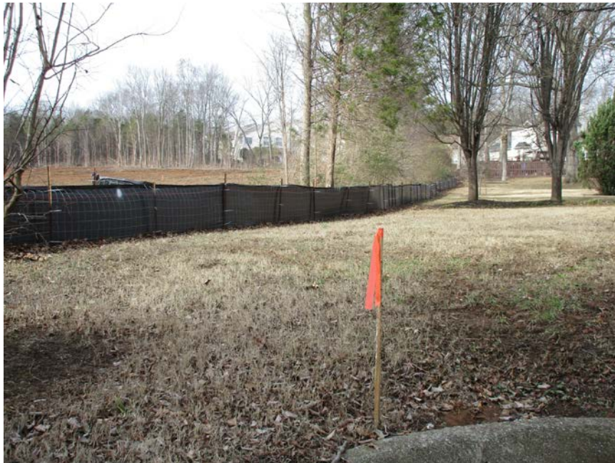
Figure 5. TDH photograph of a survey flag at the concrete curb of the dead end of Forest Pointe Place showing conditions of the cleared site, erosion control fencing, and backyard areas of several homes along the southwest side of Forest Pointe Place taken January 16, 2017. Survey flag was assumed to be the eastern property line that runs southeast to northwest.
