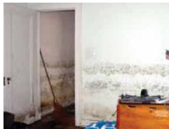
PHOTO: Mold growth in flooded home.
