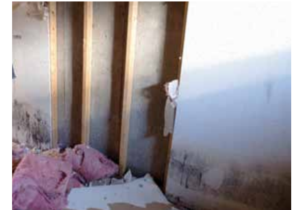
PHOTO: Remove all wet or fire-damaged insulation, even if wallboard appears to have dried.
