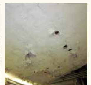
PHOTO 2: Ceiling damage resulting from roof leaks.
