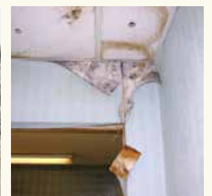
PHOTO 4: Mold behind vinyl wallpaper.
