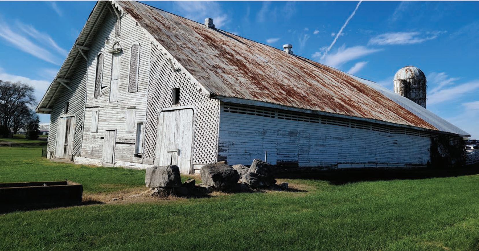
This intricately detailed barn is located on the National Register-listed Haynes Haven Stock Farm in Maury County, Tennessee. Constructed in 1890, the interior of the barn features a central aisle flanked by drive-through side bays. The exterior is covered in wood weatherboard and lattice detailing, with bargeboard detailing adorning the barn roofline. This combination of function and detail makes for a striking barn. The nomination for the property was approved by the National Park Service on July 6, 2023. Photograph courtesy of Tegan Baiocchi, November 15, 2022.
