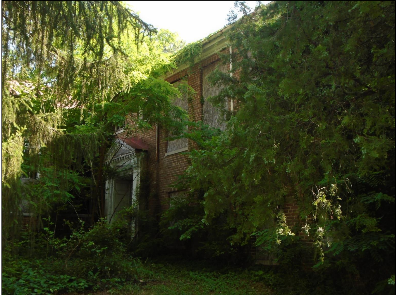
Figure 3: Entry Door, located on the west elevation of the East Wing, June 2020
