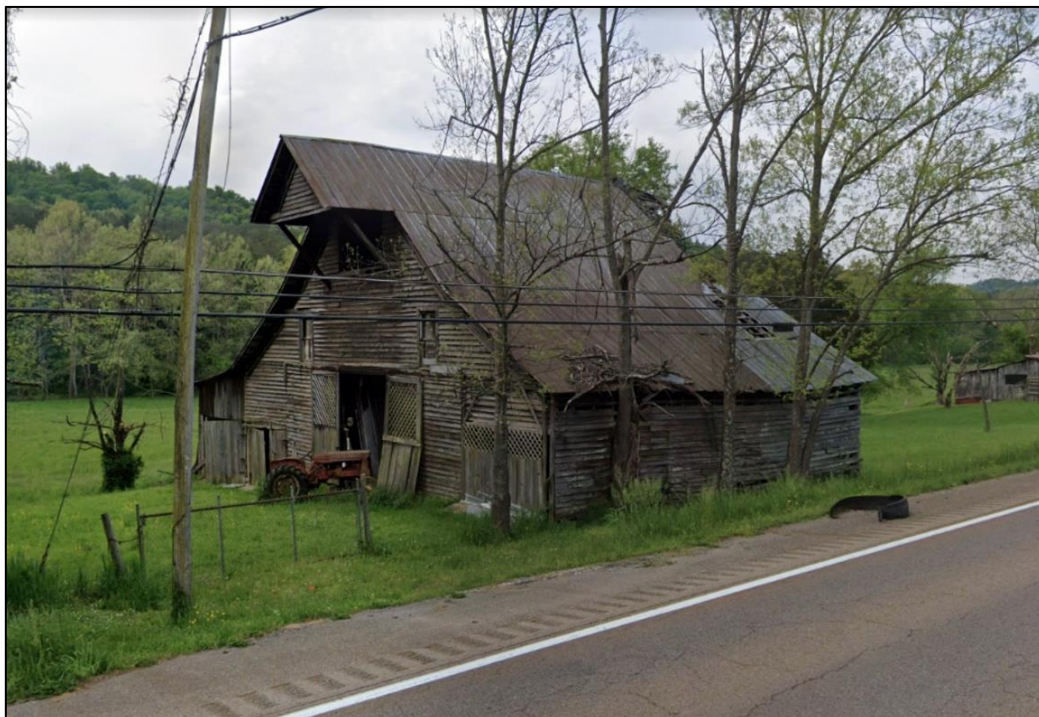
Figure 20. Feeder Barn, Rutledge Pike, Grainger County, Tennessee. Courtesy of Google Street View, April 2018.
