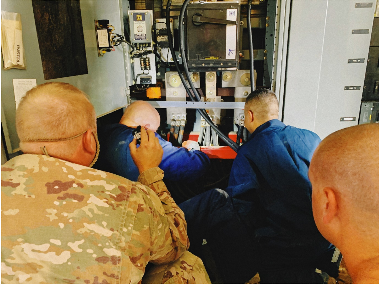
Members of the 118th Civil Engineer Squadron prepare to attach generator power to the Army National Guard Armory on Holtzclaw Avenue in Chattanooga on August 7 as part of Vigilant Guard 2021 exercise. (Photo by Lt. Col. Marty Malone)
