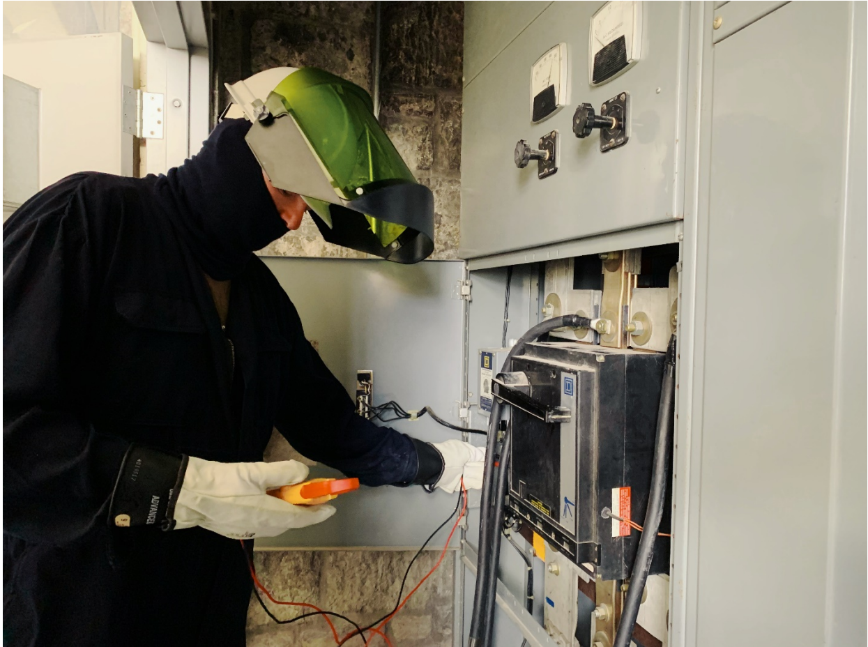
Staff Sgt. Robert Moore, working in electrical protective gear, tests electric power provided by generators from the 118th Civil Engineer Squadron as it powers the Army National Guard Armory in Chattanooga. (Photo by Lt. Col. Marty Malone)
