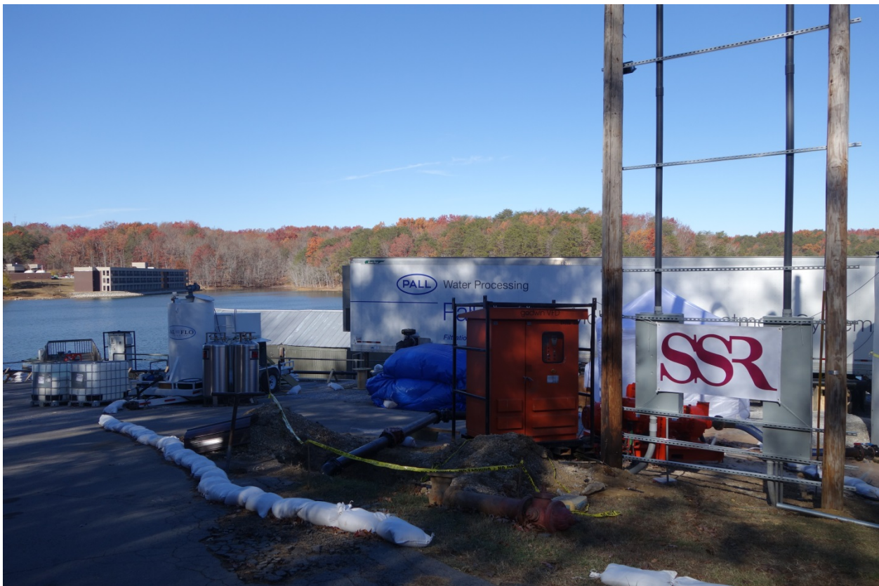
Emergency WTP at Fall Creek Falls State Park Marina
