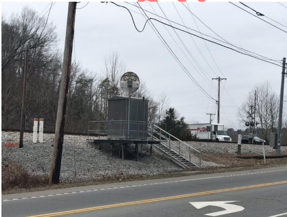
Signal Control Box 2 Panel, located at HWY 70
