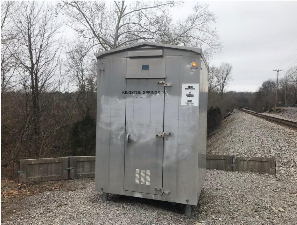
Signal Control Box 1 Panel, located at E Kingston Spring Rd
