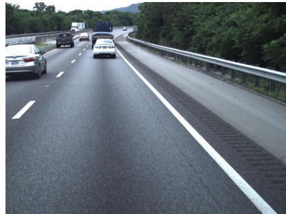
Shoulder only partially overlaid with OGFC
