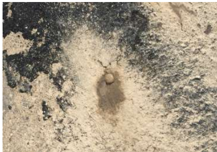
Saturated subbase that pumps, causing expensive base failures
