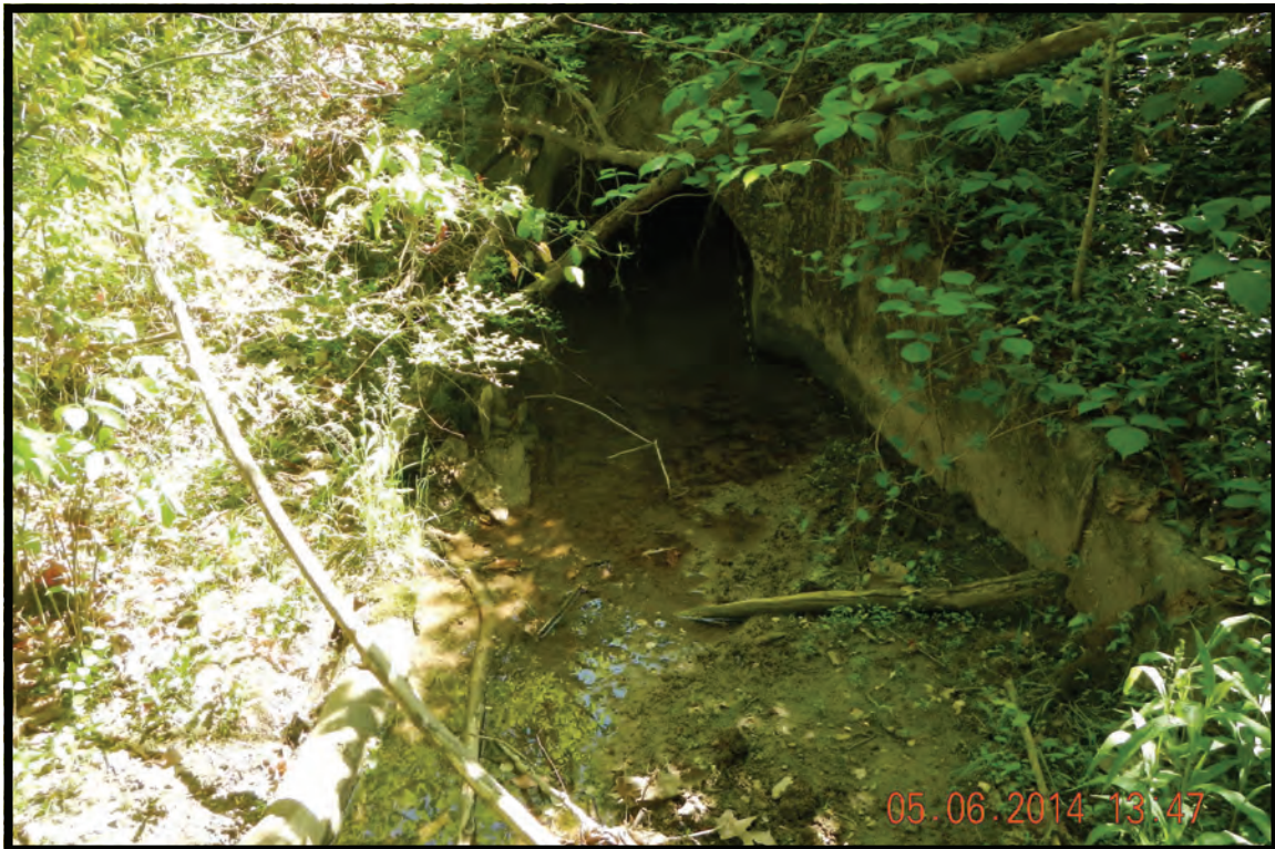
Photo 14 (3124): (Alternative D) View of STR-3 culvert on the west side of Sam Houston School Road.
