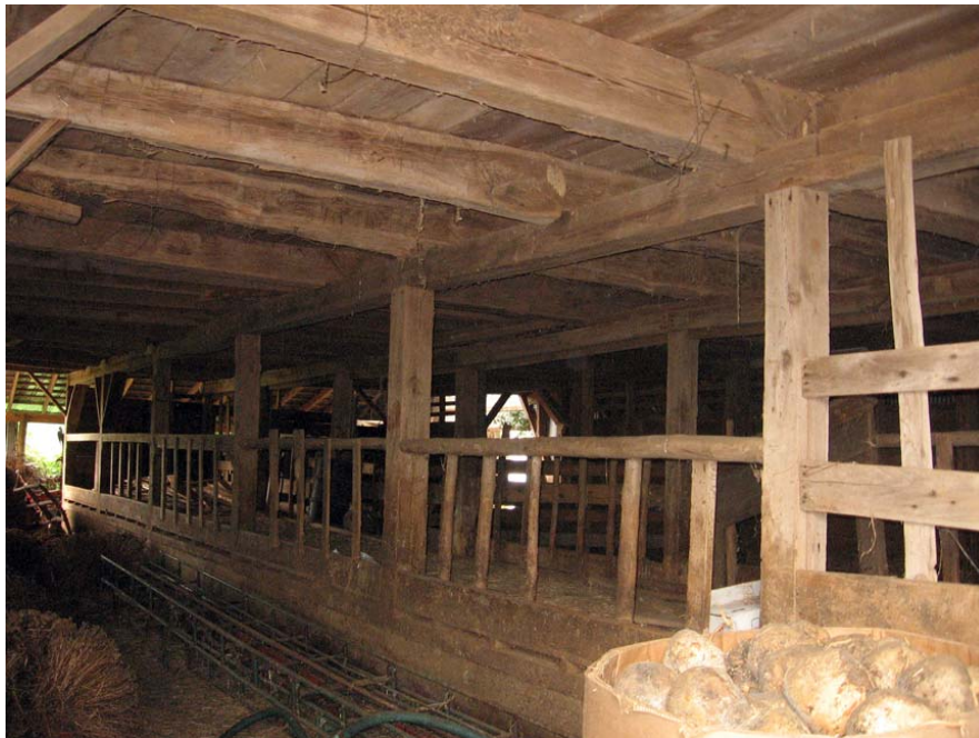
Figure 160. Chandler-DeLozier Farm looking southeast at the interior of the original cattle barn (BT.2441); note the cantilevered structural timbers, which taper toward the end in similar fashion to log cantilever barns (R. Jones 9/9/08).
