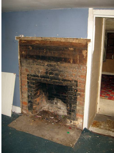
Figure 133. Clyde Irwin House, looking at the west room fireplace with is missing mantel (R. Jones 9/10/08)
