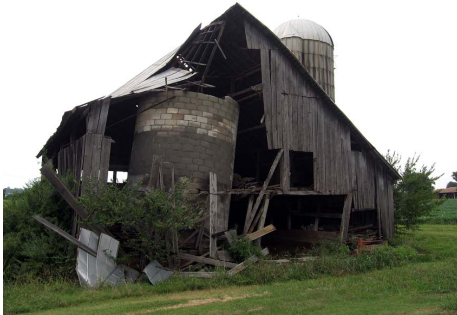
Figure 158. Chandler-DeLozier Farm looking west at the dairy barn (BT.2442) built by George Chandler in the 1920s or '30s; the concrete block grain silo is leaning due to a failing foundation (R. Jones 9/9/08).
