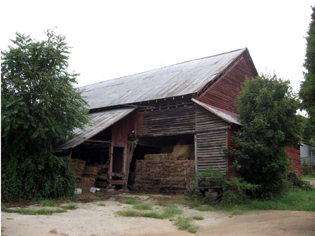
Figure 159. Chandler-DeLozier Farm looking southeast at the original cattle barn (BT.2441) built like a cantilever barn but without log cribs (R. Jones 9/9/08)
