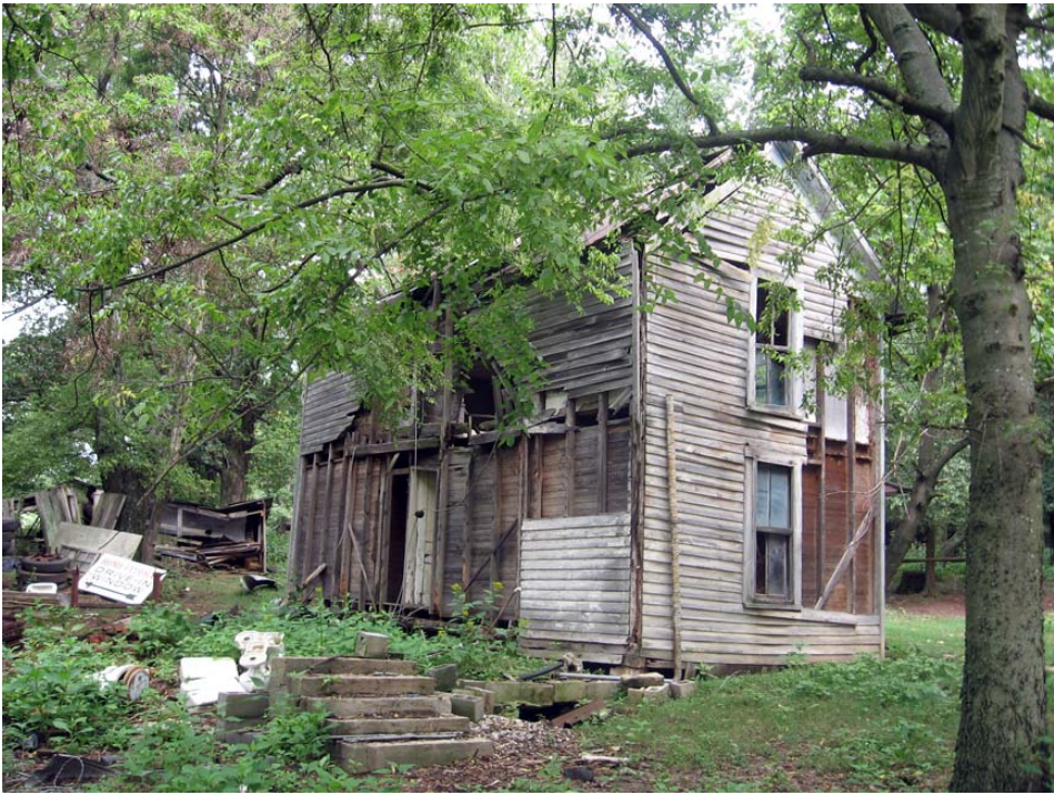
Figure 80. Ammons-Mobley Farm looking northeast at the ca. 1900 farmhouse and the now missing ca. 1880 rear ell (R. Jones 9/10/08)
