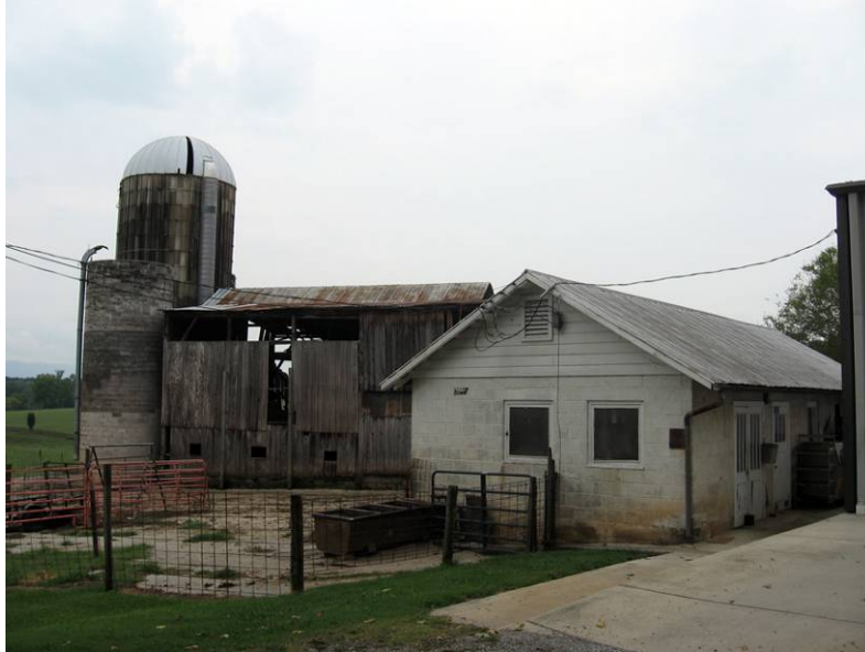
Figure 42. The Martin-Walters Farm looking southwest at the cattle barn and silos (left) and Bulk Milk Cooler (right) (R. Jones 9/9/08)
