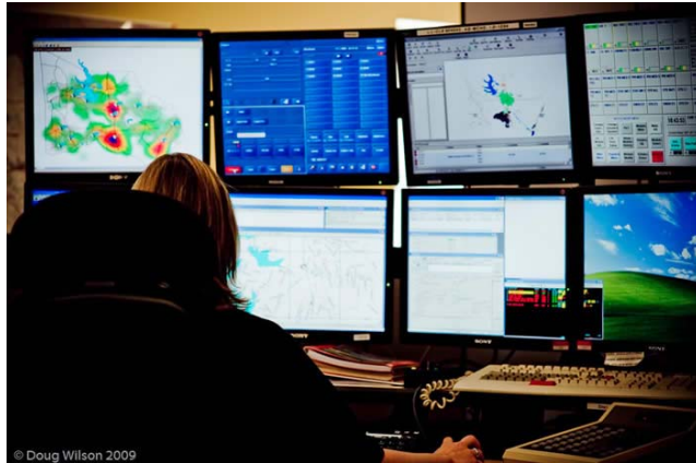
Computer-Aided Dispatch Systems
