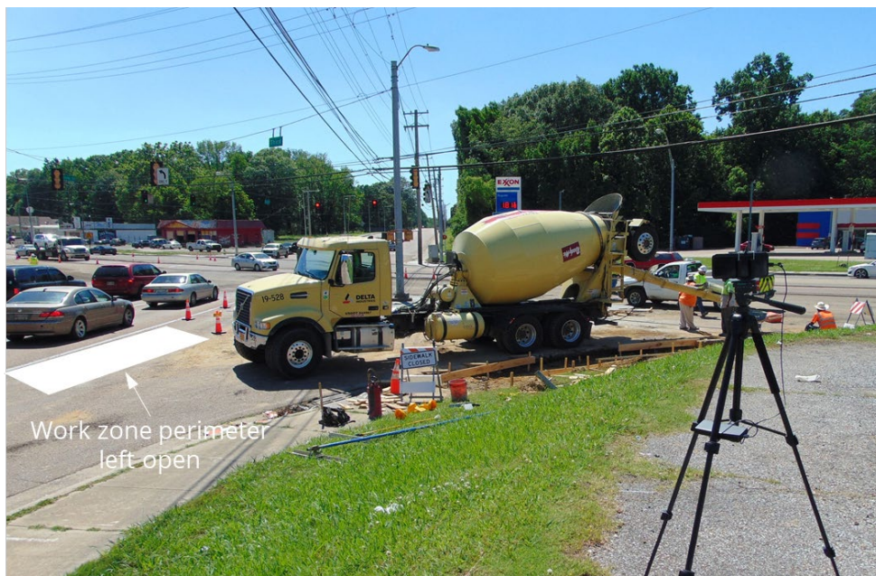
Figure 4-34. Project 5: Work zone perimeter left open
