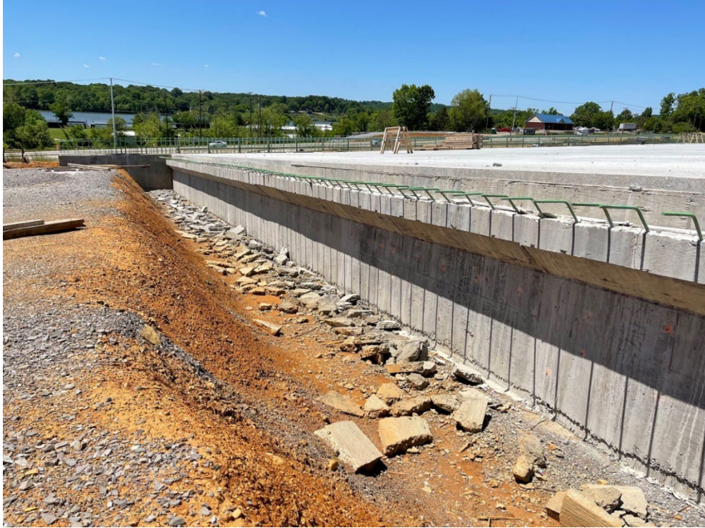
Figure 3-2. Photo of the face of the south abutment before constructing the approach slab.
