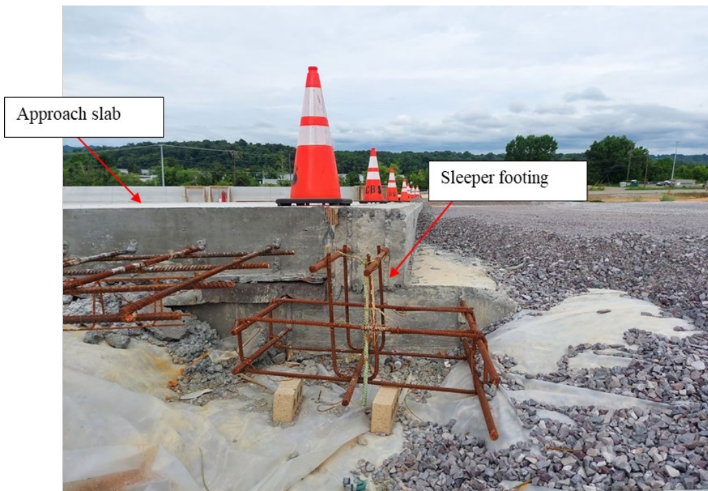
Figure 3-5: Side view of the north approach slab and sleeper footing. A new lane was added to the bridge after this project ended.
