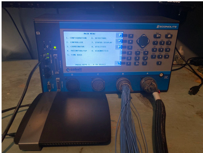
Figure 5.1 The test setup of the Econolite Cobalt Traffic Signal Controller
