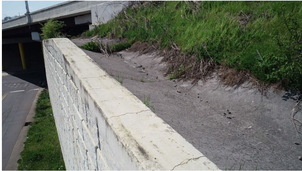
Figure A. 3 Cracks observed on top of the wall, clear drainage path on top of the wall
