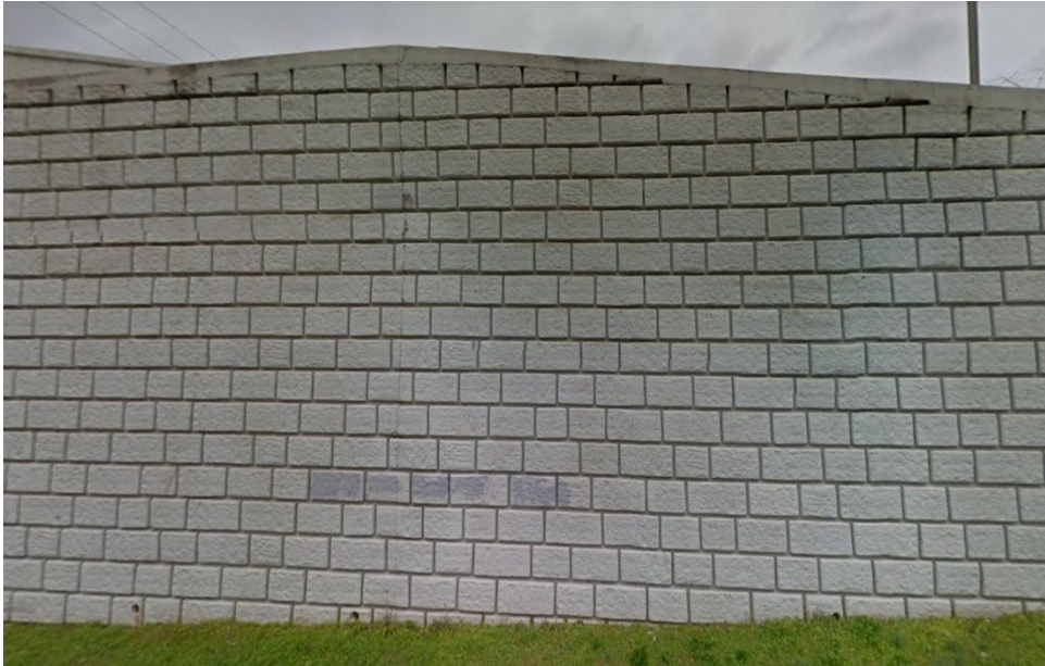
Figure A. 1 Vertical crack on wall facing
