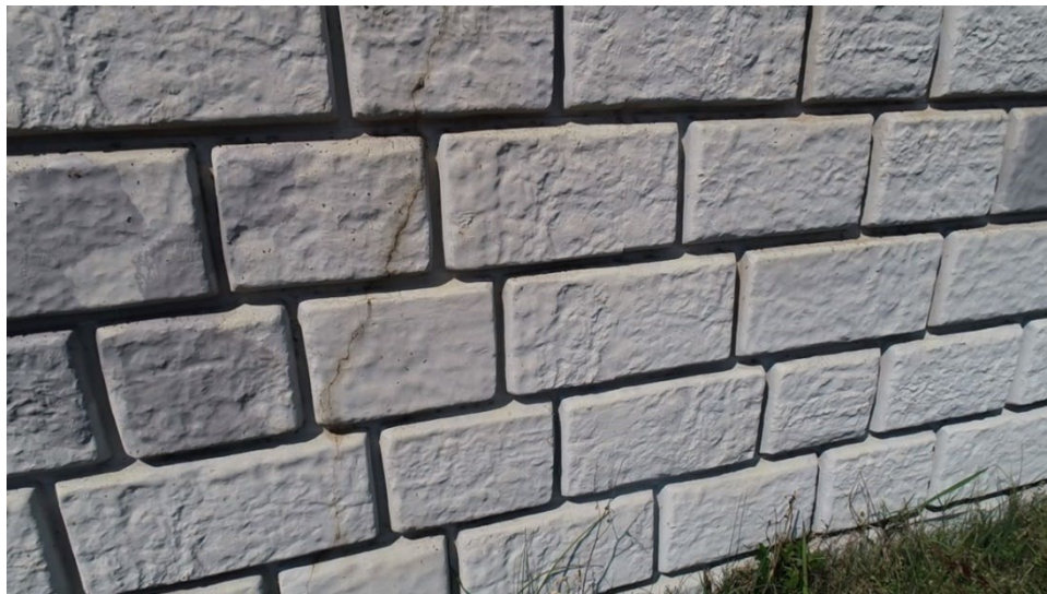
Figure A. 6 Moderate cracks observed on the face of the wall blocks
