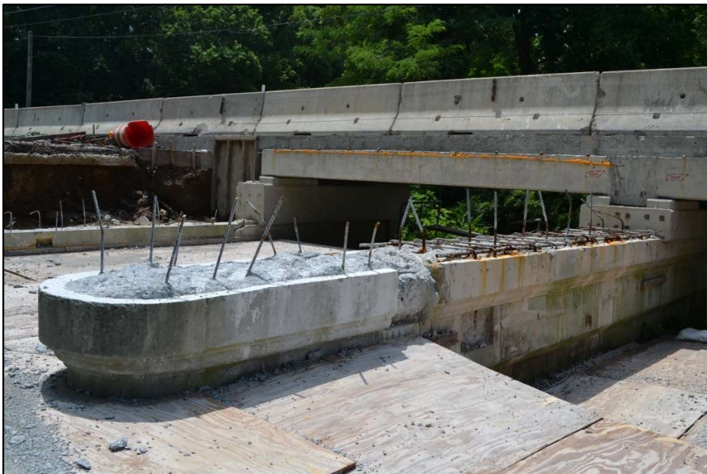
Figure 4-14: Substructure – Partially Repaired
