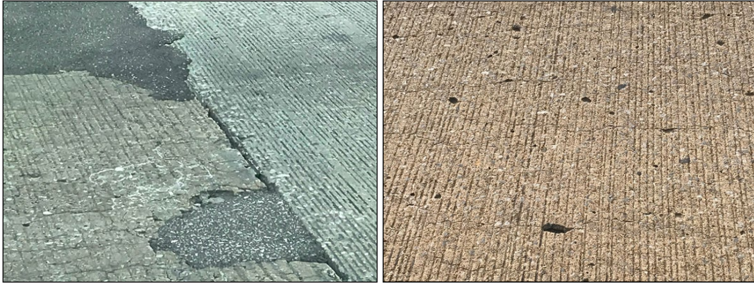
Figure C- 3 Cracking of a concrete pavement in Memphis, TN (Photo credit: Derek Gaw-TDOT)
