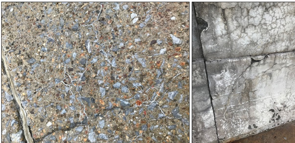
Figure C- 2 Cracking in concrete pavement and barrier wall in Flag Pond, TN (Photo credit: Derek Gaw-TDOT)
