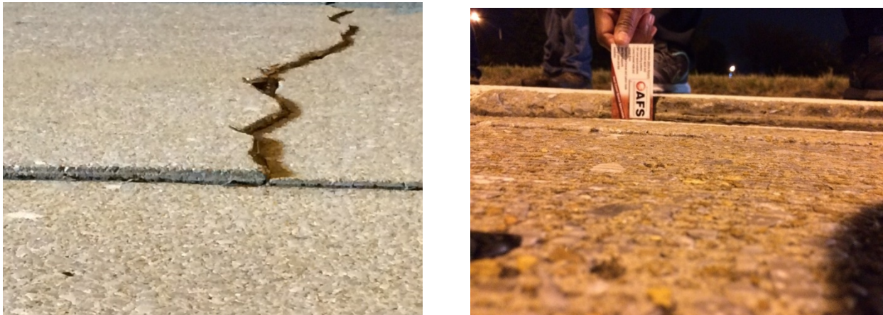
Figure 1.2 Mid slab cracks and longitudinal joint faulting of over 1 in. on I-24 West
