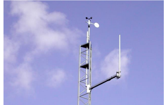
Figure 21. TDOT weather sensor
