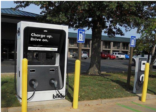
Figure 23. Electric Vehicle Charging Station at Cracker Barrel in Lebanon, TN
