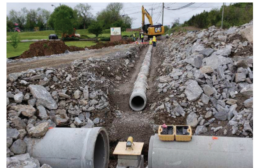
Storm drain installation and preparation for catch basin location near the YMCA.
