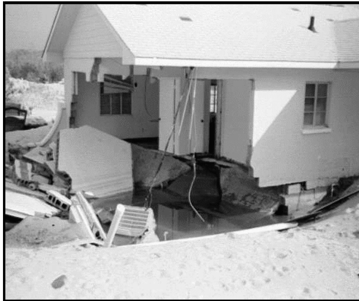
Figure 1-16. Beaches are particularly susceptible to undermining of foundations due to velocity flows.
